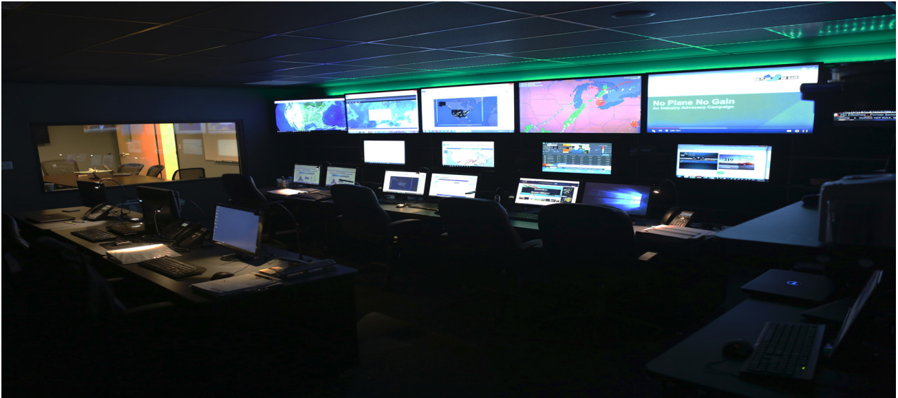
Fireside's Emergency Operations Center
